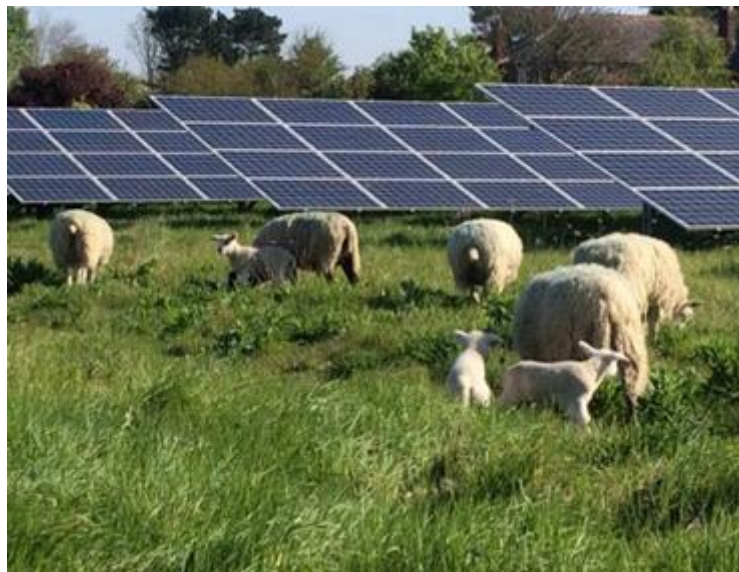
Above: Typical solar panels and mounting
