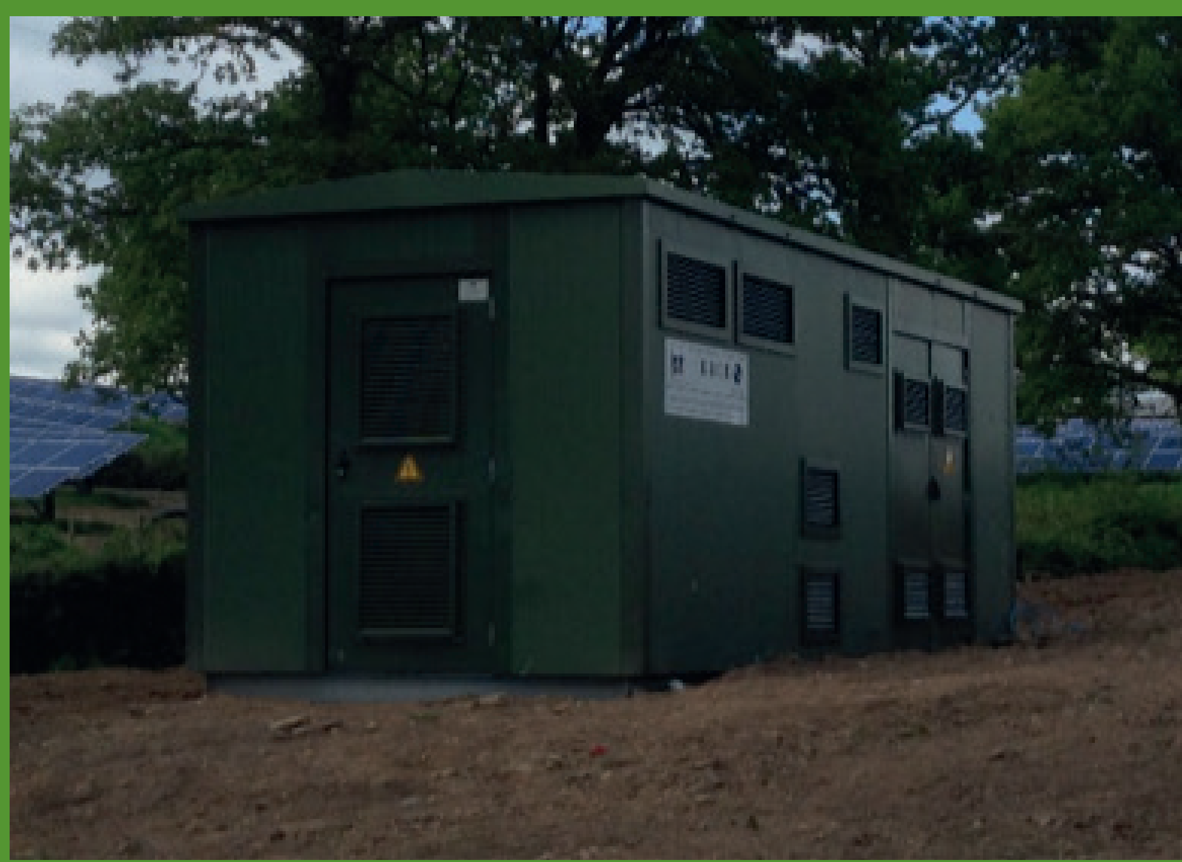
Typical Site Substation
