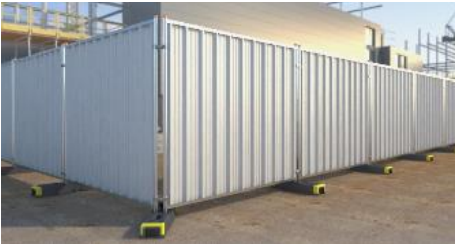
Figure 5.1 Example Metal Hoarding
