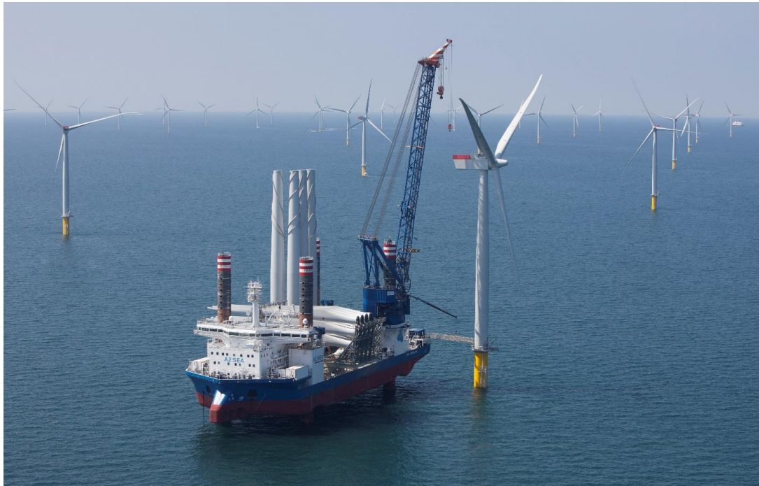
Plate 2.5 Wind Turbine under Construction (photo taken from West of Duddon Sands offshore windfarm)
