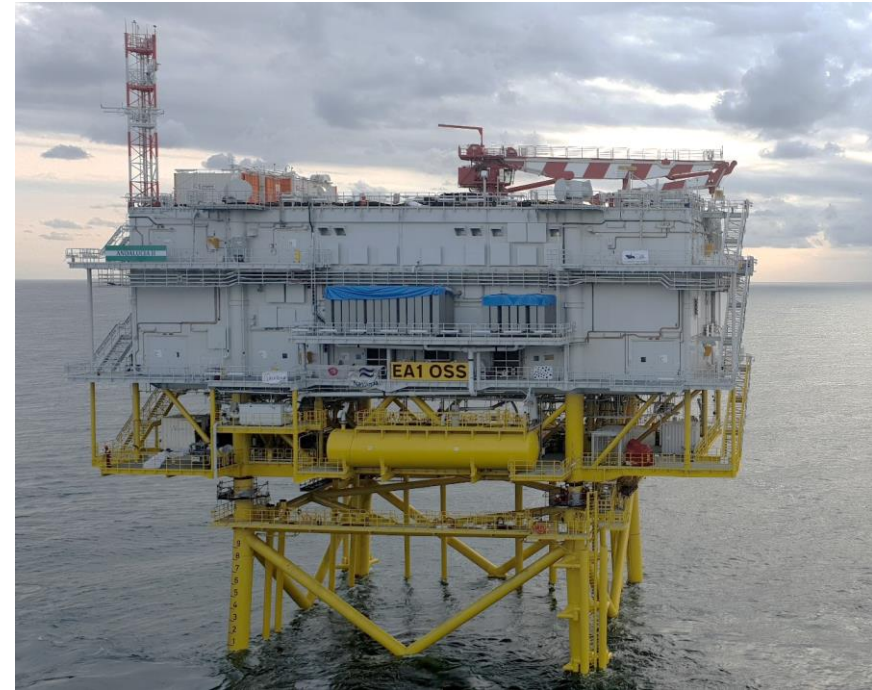
Plate 2.4 Offshore Electrical Platform
