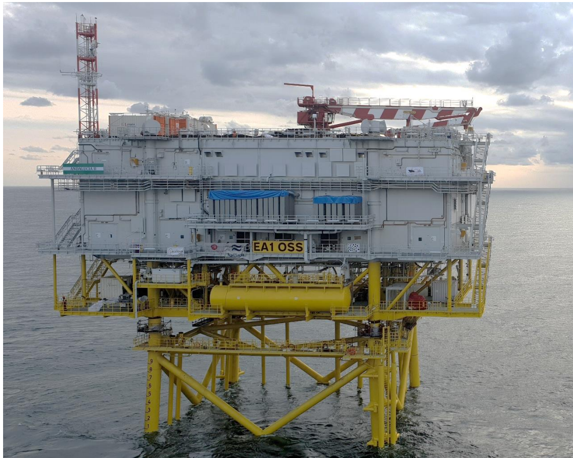
Plate 6.7 Typical offshore electrical platform (AC collector station) (SPR 2018)
