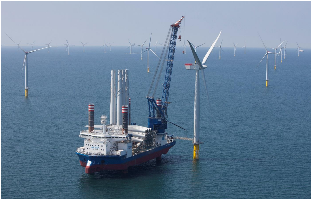
Plate 6.9 Wind Turbine under Construction (photo taken from West of Duddon Sands offshore windfarm)
